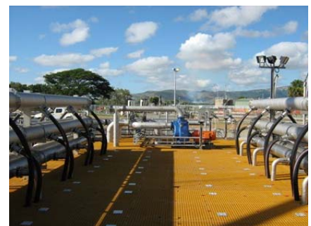
Figure 3: Permeate & Air Pipes on MBR
