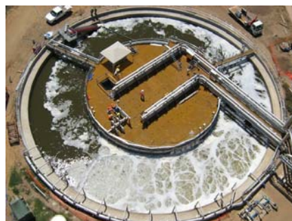
Figure 2: Clarifier Converted into MBR
