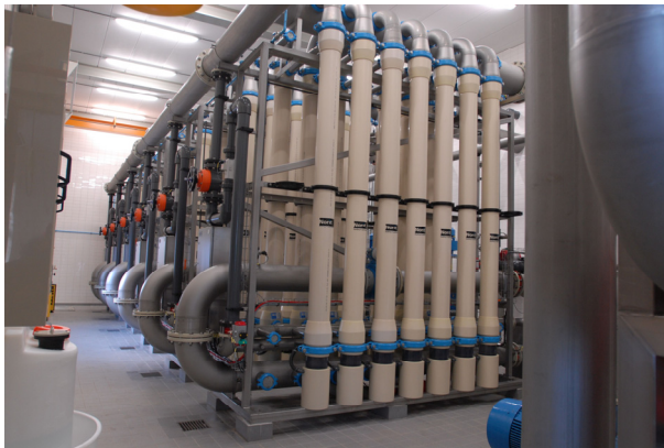
Figure 2. Full-scale side-stream Airlift MBR system for municipal waste water treatment.
