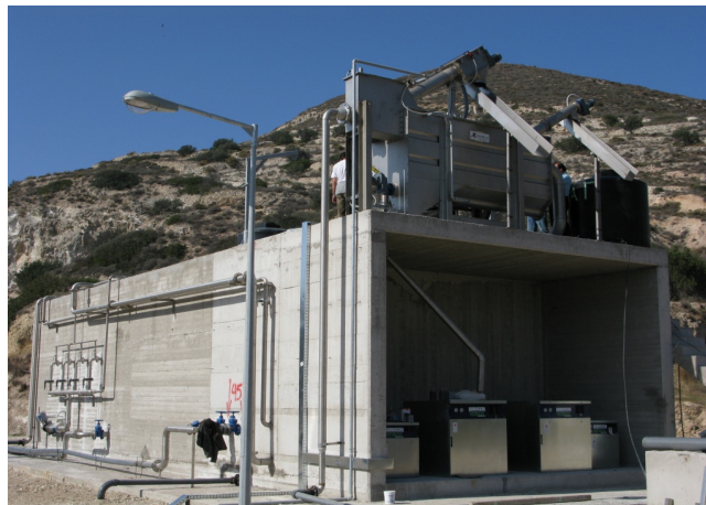
Plate 2: View of the plant main structure, including fine screening/grit removal, de-nitrification tank and membrane tanks, during commissioning (Kubota Corporation).
