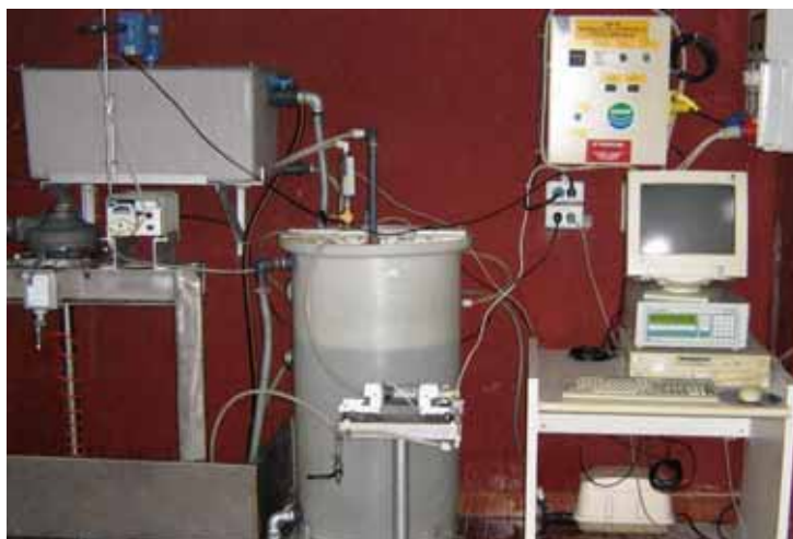
Figure 1 - MBR pilot plant installed in Milano Nosedo WWTP.
